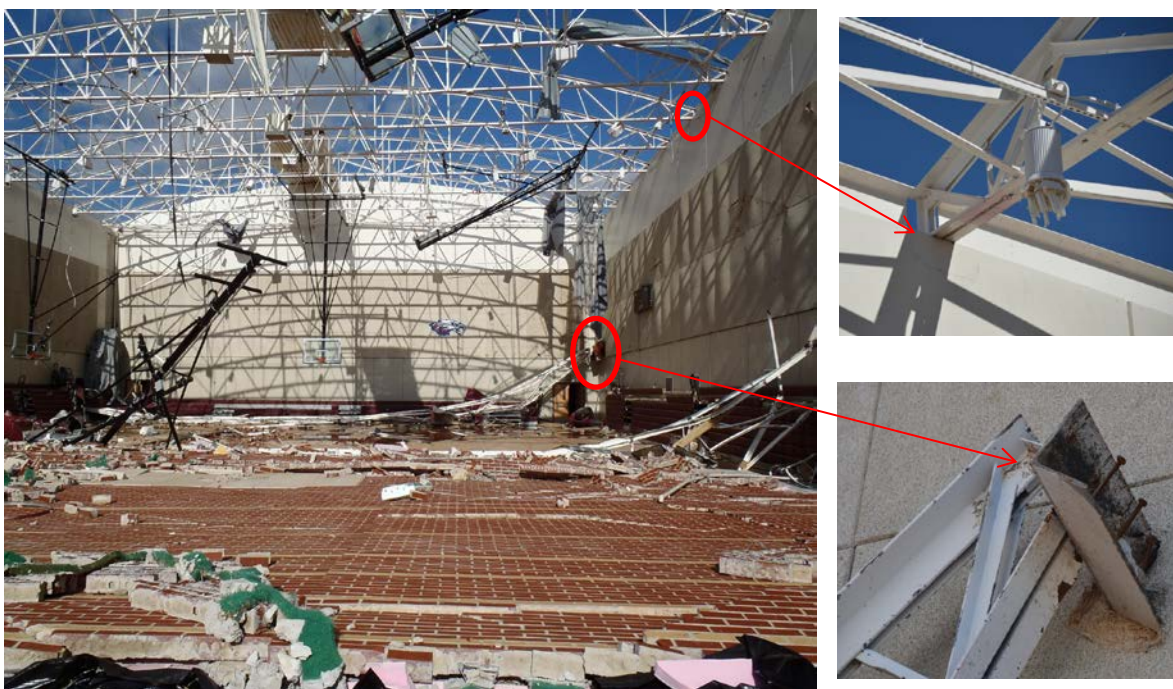
Figure 4. Example of photographic field data used in developing a failure hypothesis for the gymnasium at Joplin East Middle School. (Photo source: NIST)
