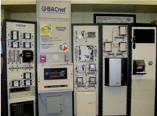
Virtual Cybernetic Building Testbed Control System Hardware
