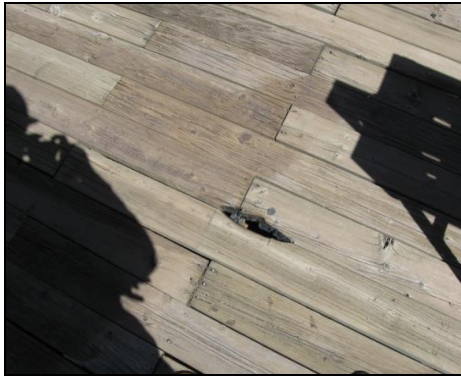
Figure 44 Ignited deck, which was extinguished by homeowners, NIST photo.
