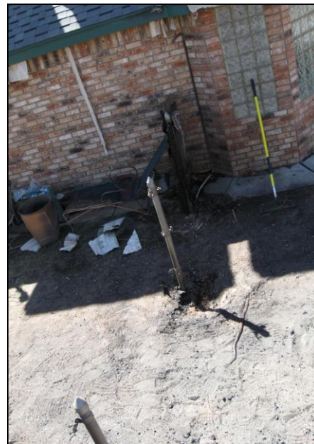
Figure 57 Partially destroyed wood fence, which caused scorching to brick siding and melting of vinyl soffit, NIST photo.
