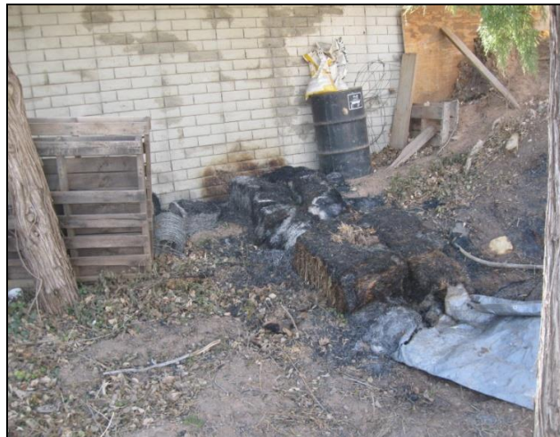
Figure 33 Burned hay bales leading from destroyed secondary structure to primary structure causing scorching on the brick siding. Categorization of defensive actions is unknown, NIST photo.
