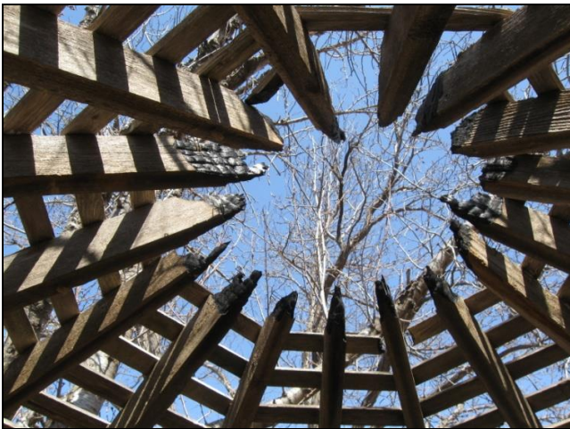
Figure 60 Damaged pergola roof ignited by embers, NIST photo.
