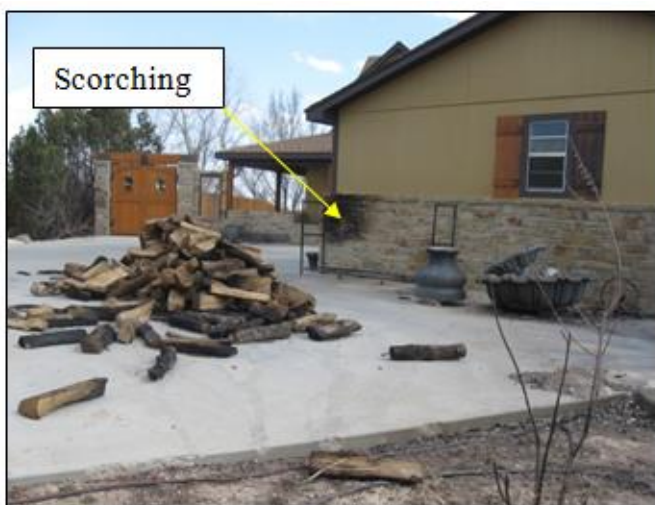
Figure 55 Defended firewood pile at 100 Camino Alto, NIST photo.
