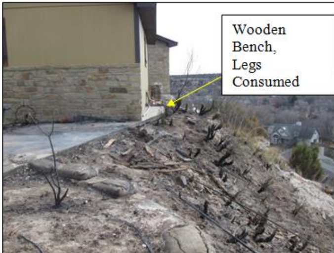
Figure 56 Damaged wooden bench and burned and unburned vegetation on west side of 100 Camino Alto, NIST photo.
