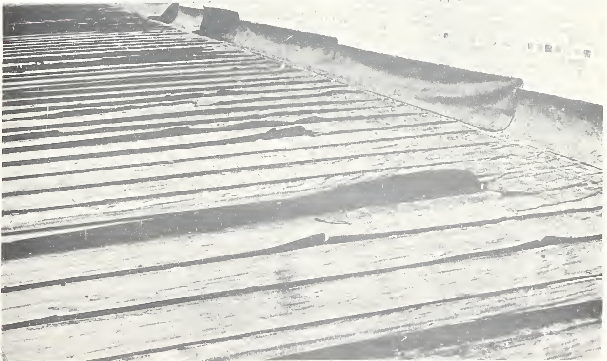
Figure 11. Leaks caused by entrance of water at defective flashings are sometimes attributed to failure of roof membrane.
