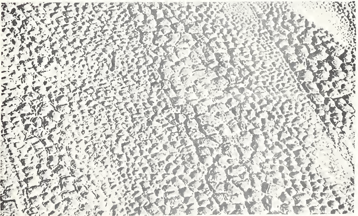
Figure 22. Alligatoring and cracking of a cold coating over alligatorated asphalt surface after one year exposure.
