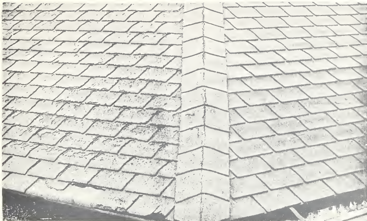
Figure 29. Differential weathering of asphalt shingles on Southern and Eastern exposures.
