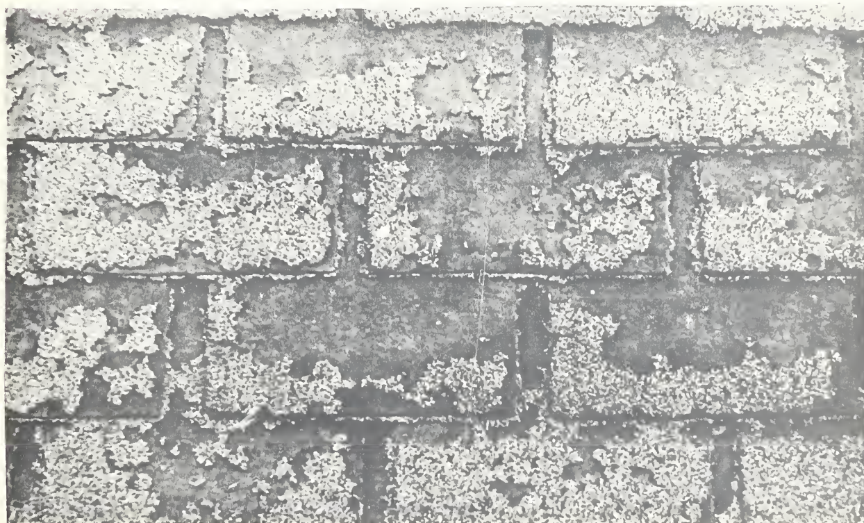
Figure 30. Severe loss of mineral granules and coating asphalt due to weathering.
