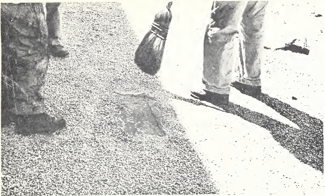
Figure 15. Insufficient bitumen to embed mineral surfacing.
