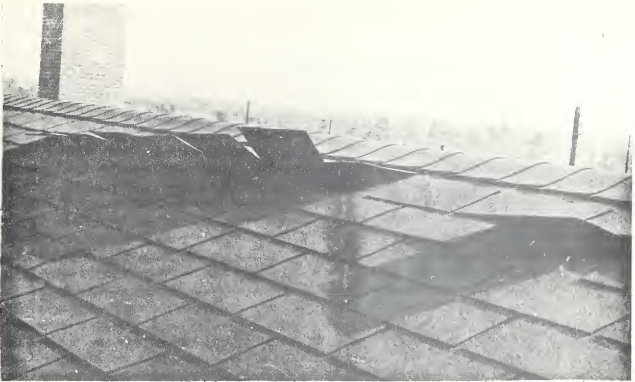
Figure 9. Action of strong winds on asphalt shingles nailed too high.
