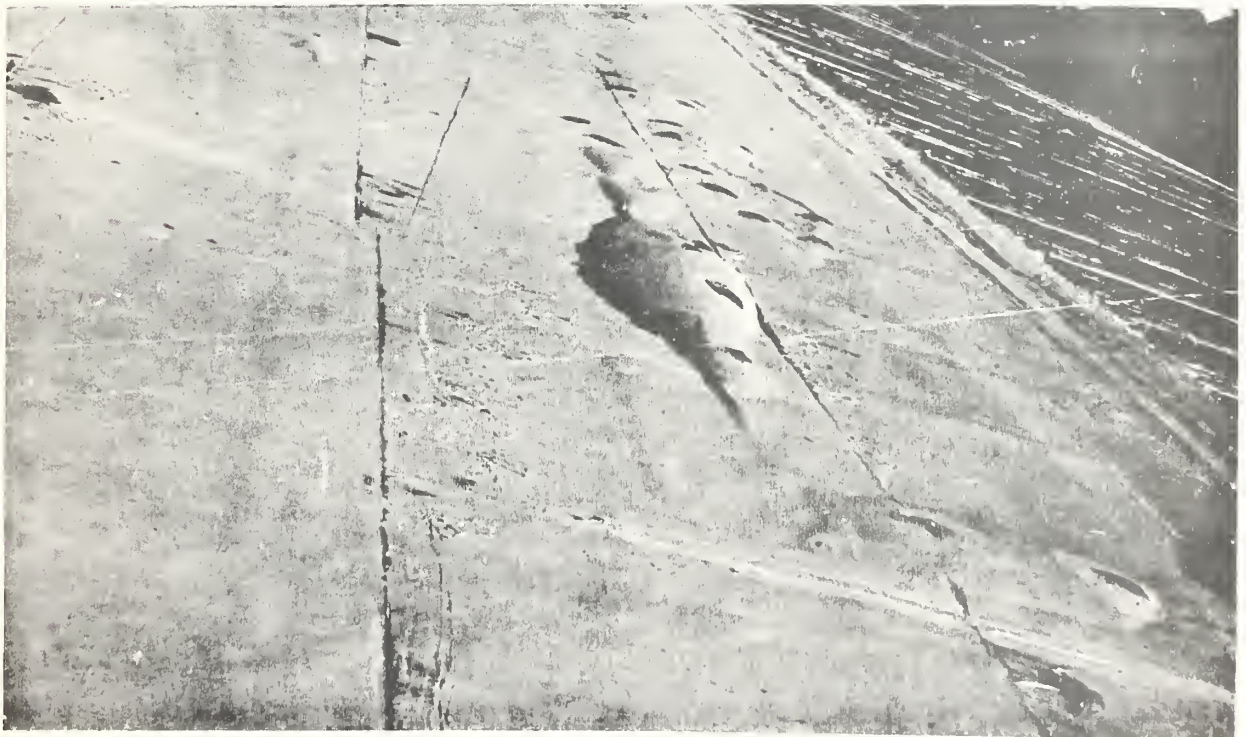
Figure 26. Large blister on smooth-surfaced roof.
