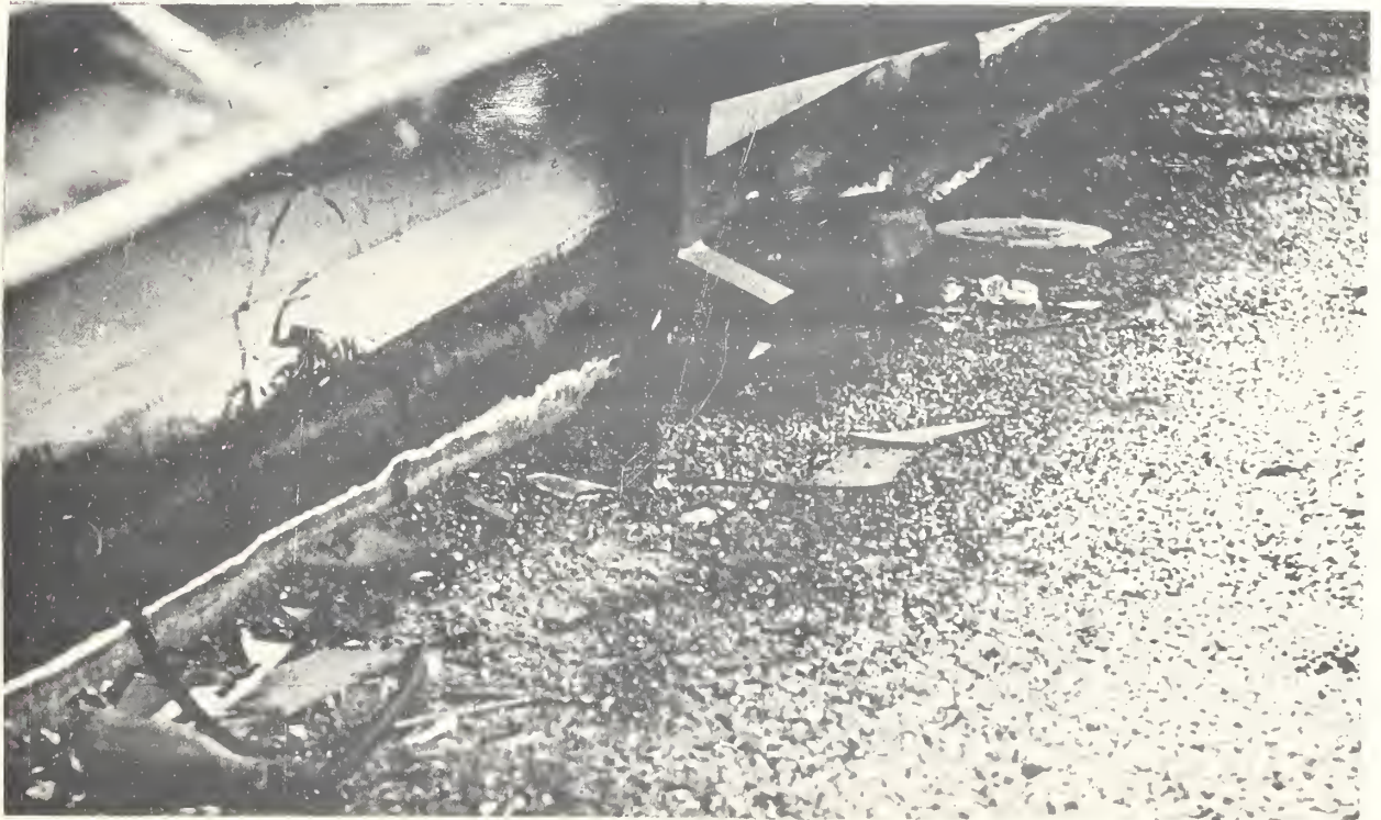
Figure 45. Debris left on roof results in poor drainage.
