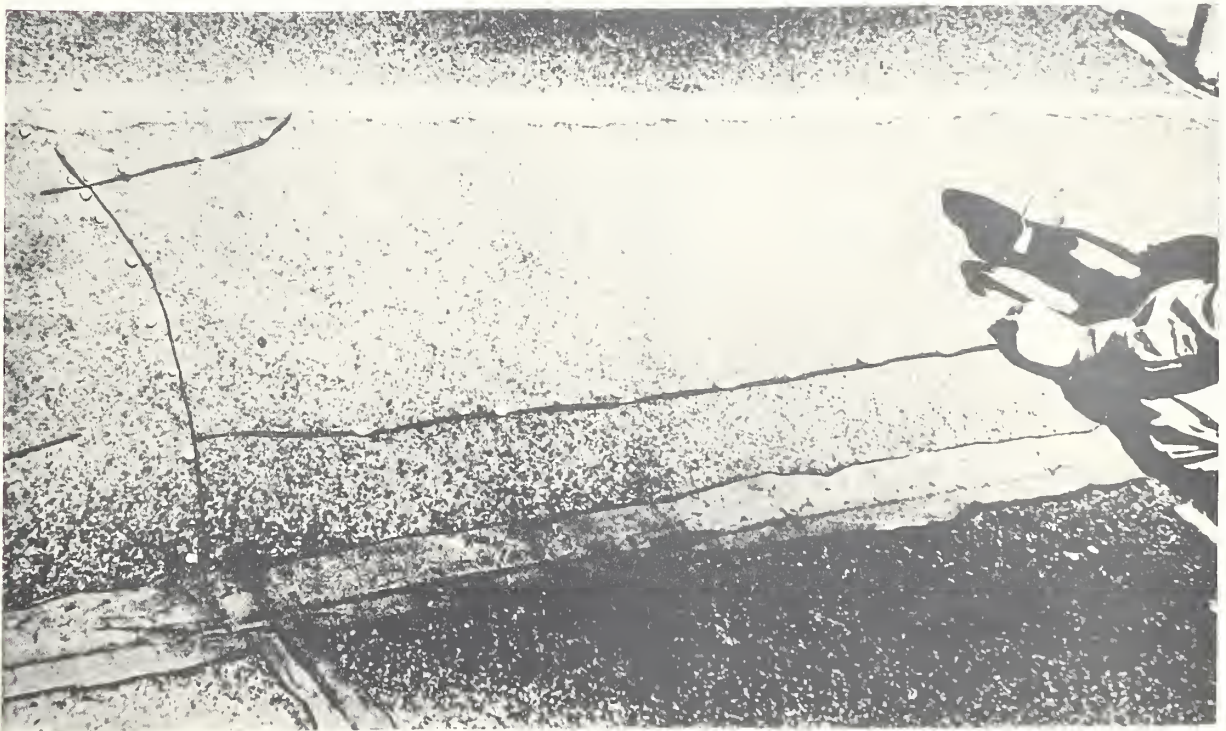
Figure 36. Buckles and wrinkles in existing roofing must be cut and edges nailed down to obtain a flat surface for application of a new roof.
