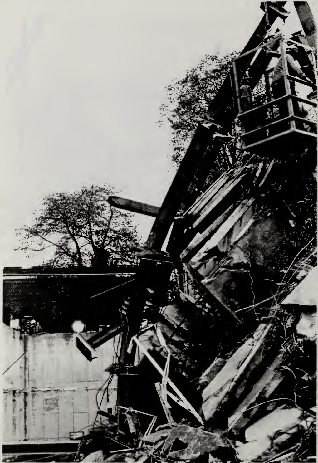
Figure 4.4.3 Deflected shape of column E1 – View to the North
