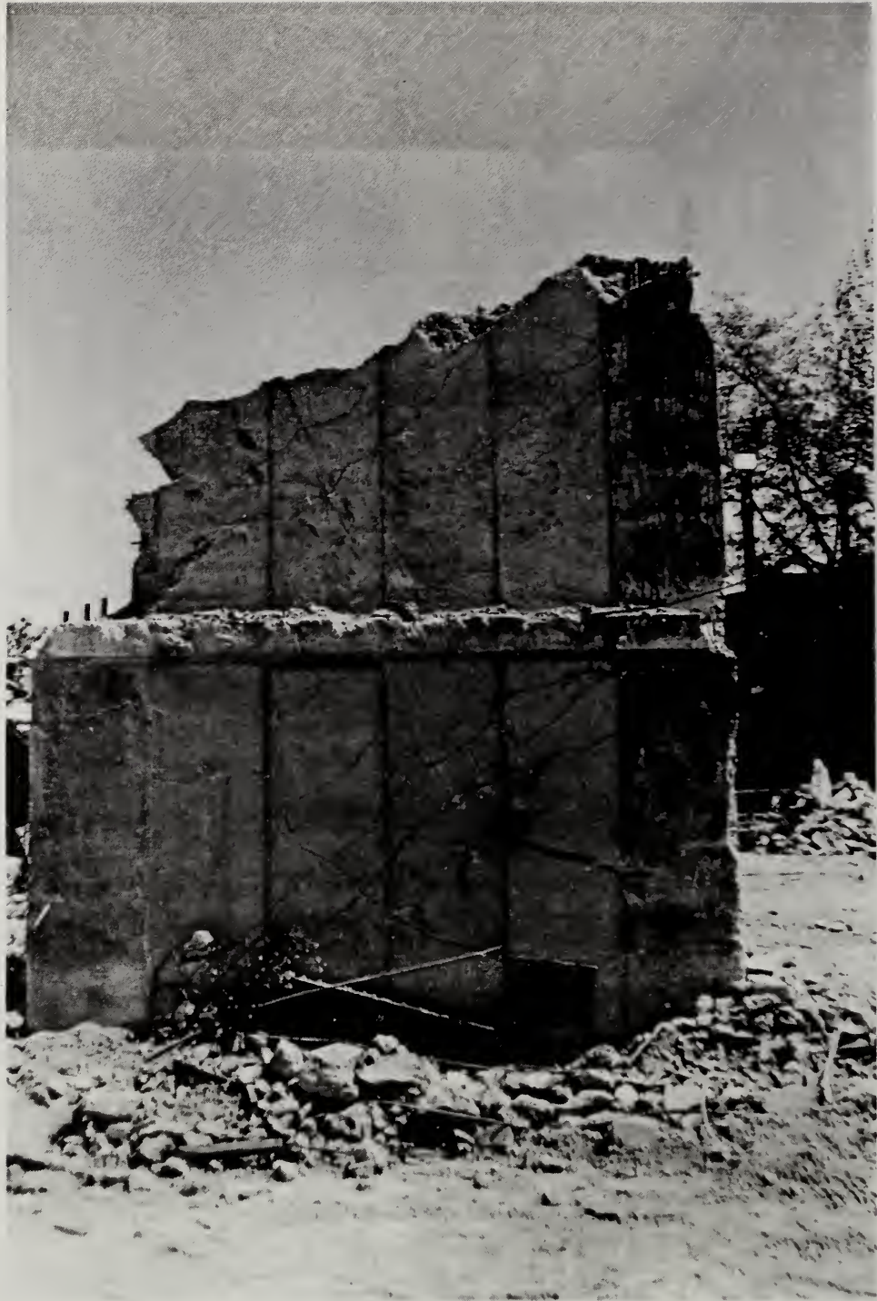
Figure 4.4.5 Diagonal tension crack in East tower shearwall - View to the South
