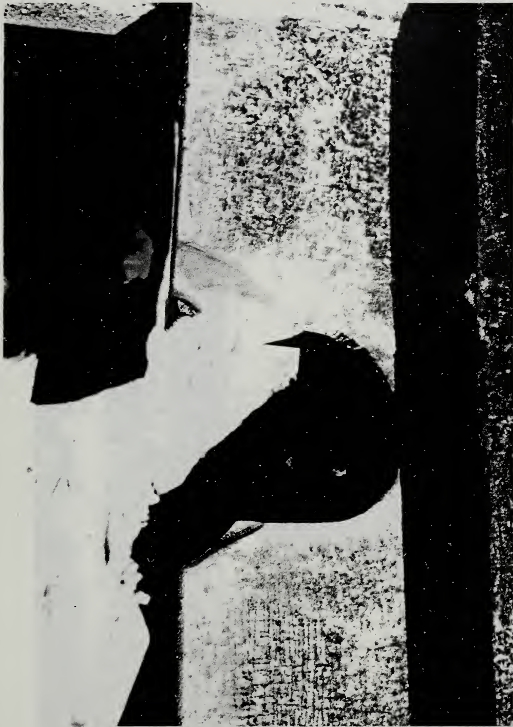
Figure 9.3.4 Indentation in underside of lifting angle, column E3.8, level 10
