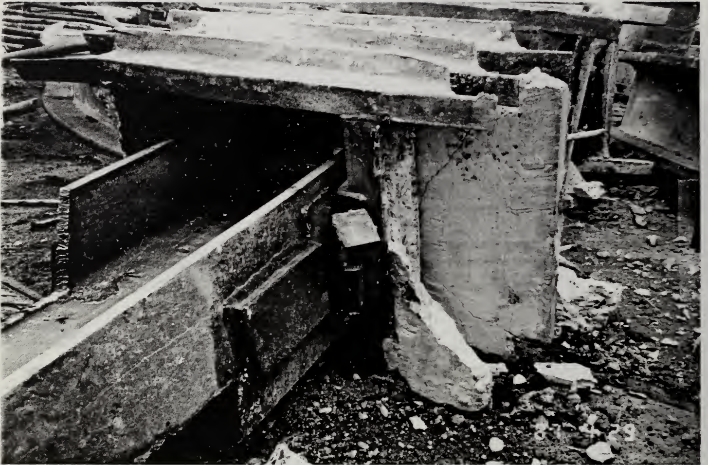
Figure 4.4.25 Weld failure at weld block with shim
