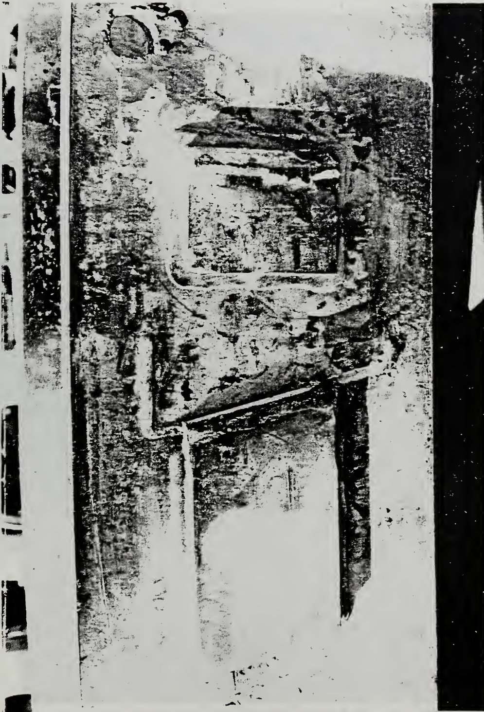
Figure 4.4.26 Weld failure at weld block
