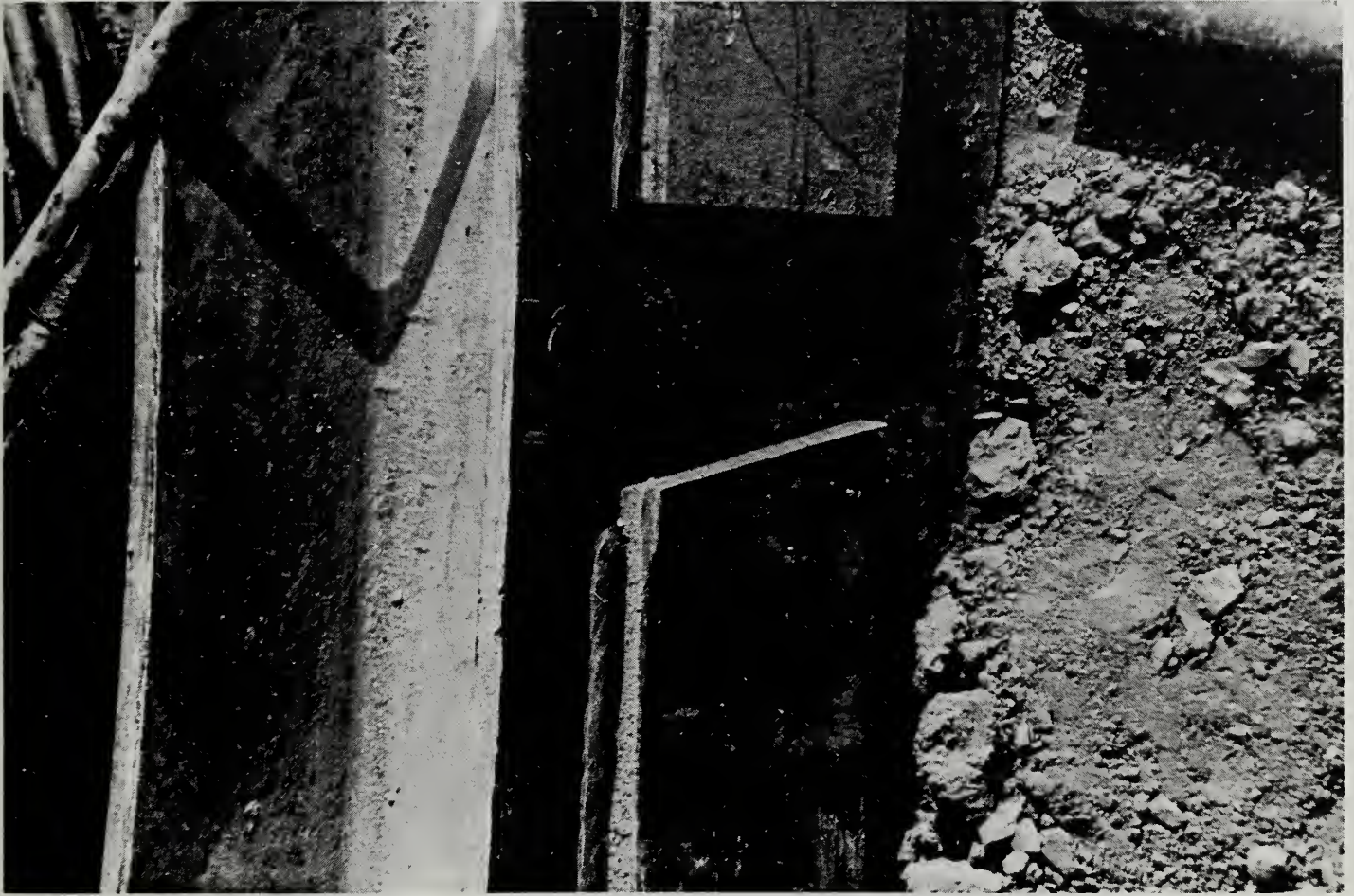
Figure 4.4.28 Failure of temporary weld at shearhead support
