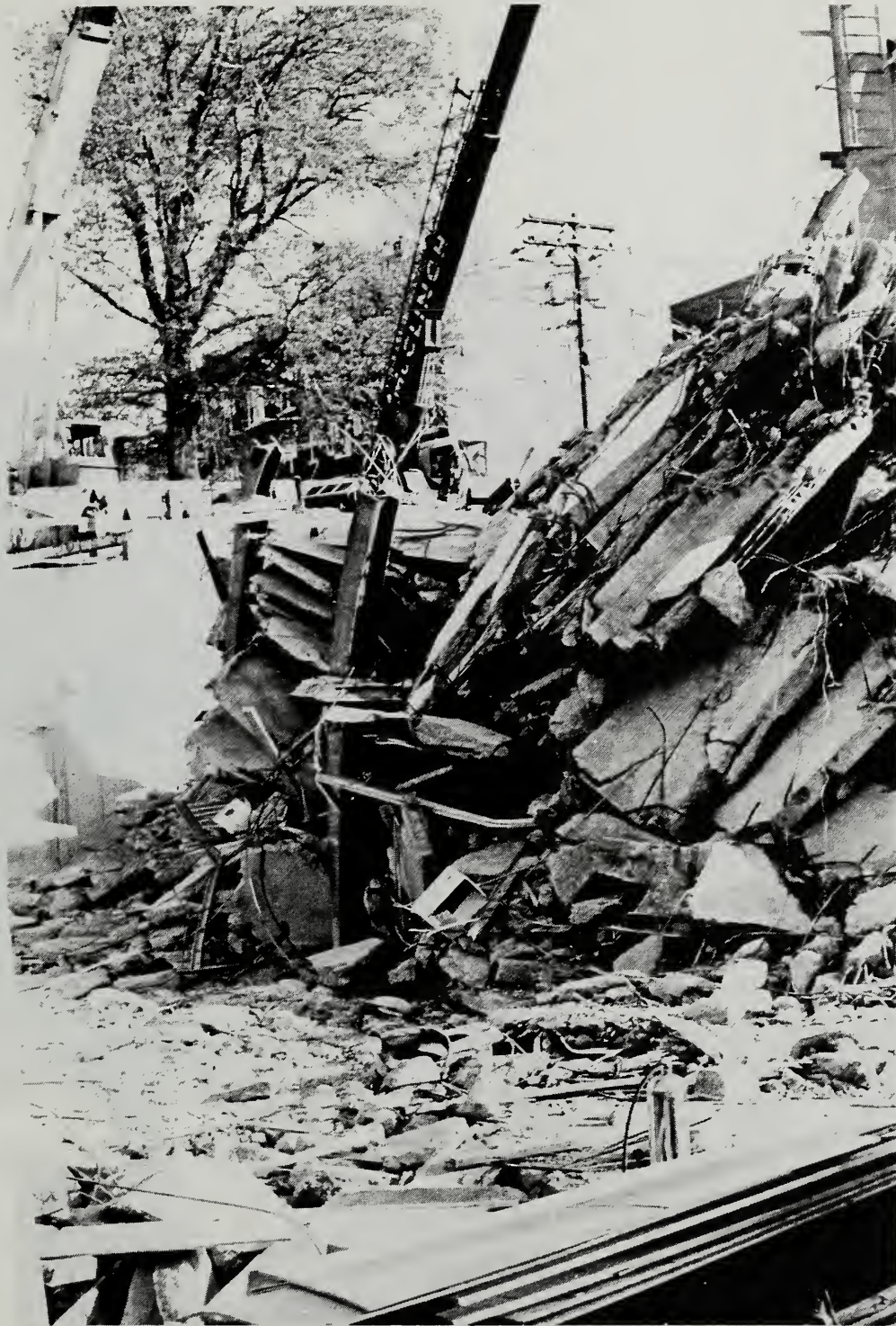
Figure 4.4.8 Lower level floor slabs at Northwest corner of West tower – View to the North; column E1
