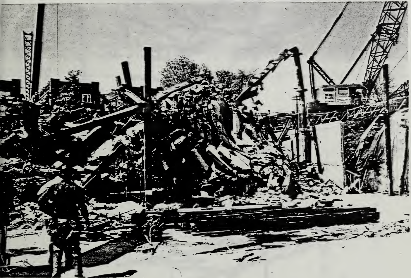
Figure 4.4.12 Floor slabs in Southeast corner of East tower - View to the Northeast
