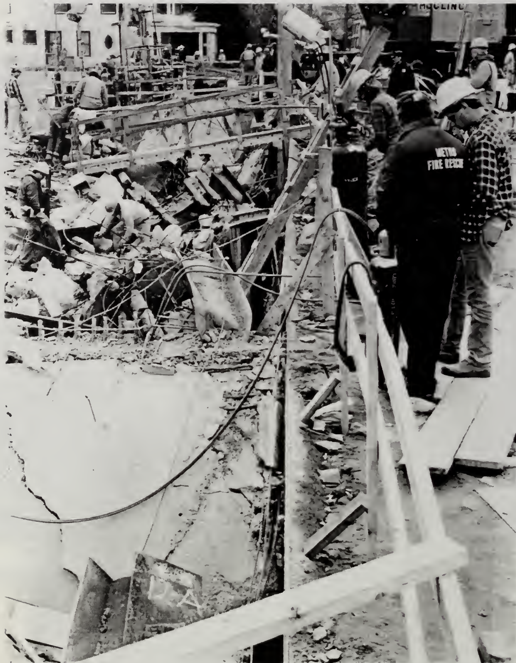
Figure 4.4.29 Basement wall on North side of East Tower – viewed from the East, May 1, 1987
