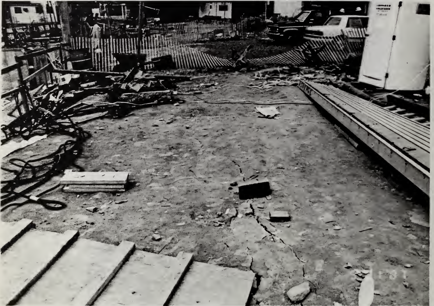
Figure 4.4.31 Tension cracks in backfill behind basement wall - North side of building
