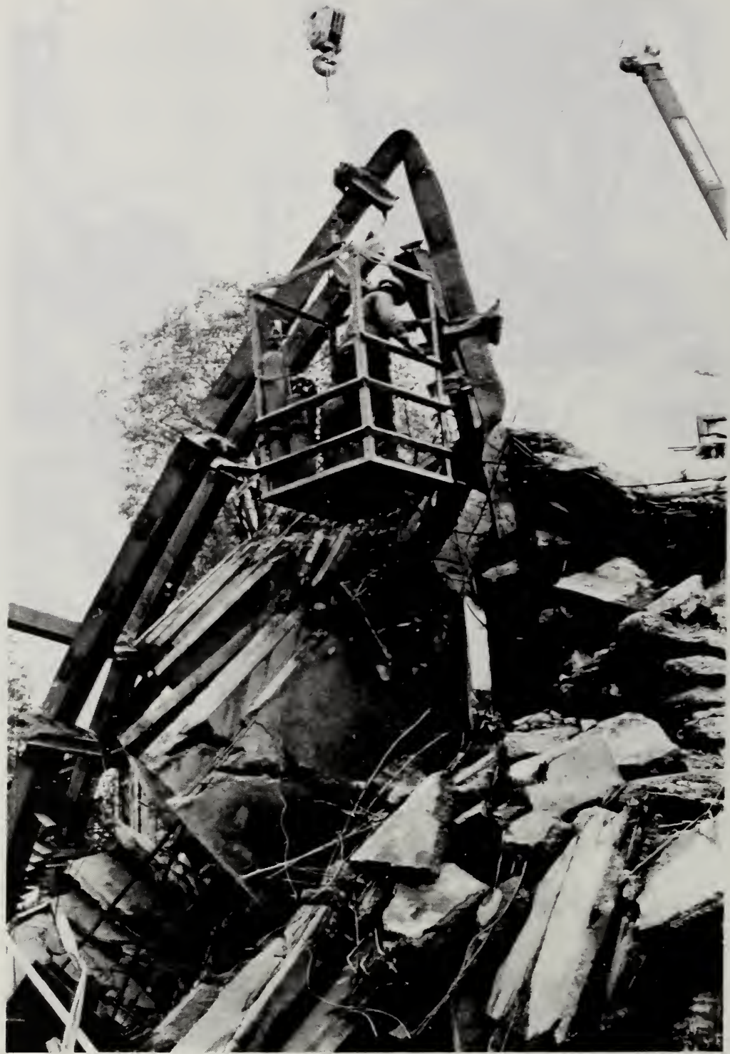
Figure 4.4.9 Upper floor slabs on Northwest corner of West tower - View to the North; column E1
