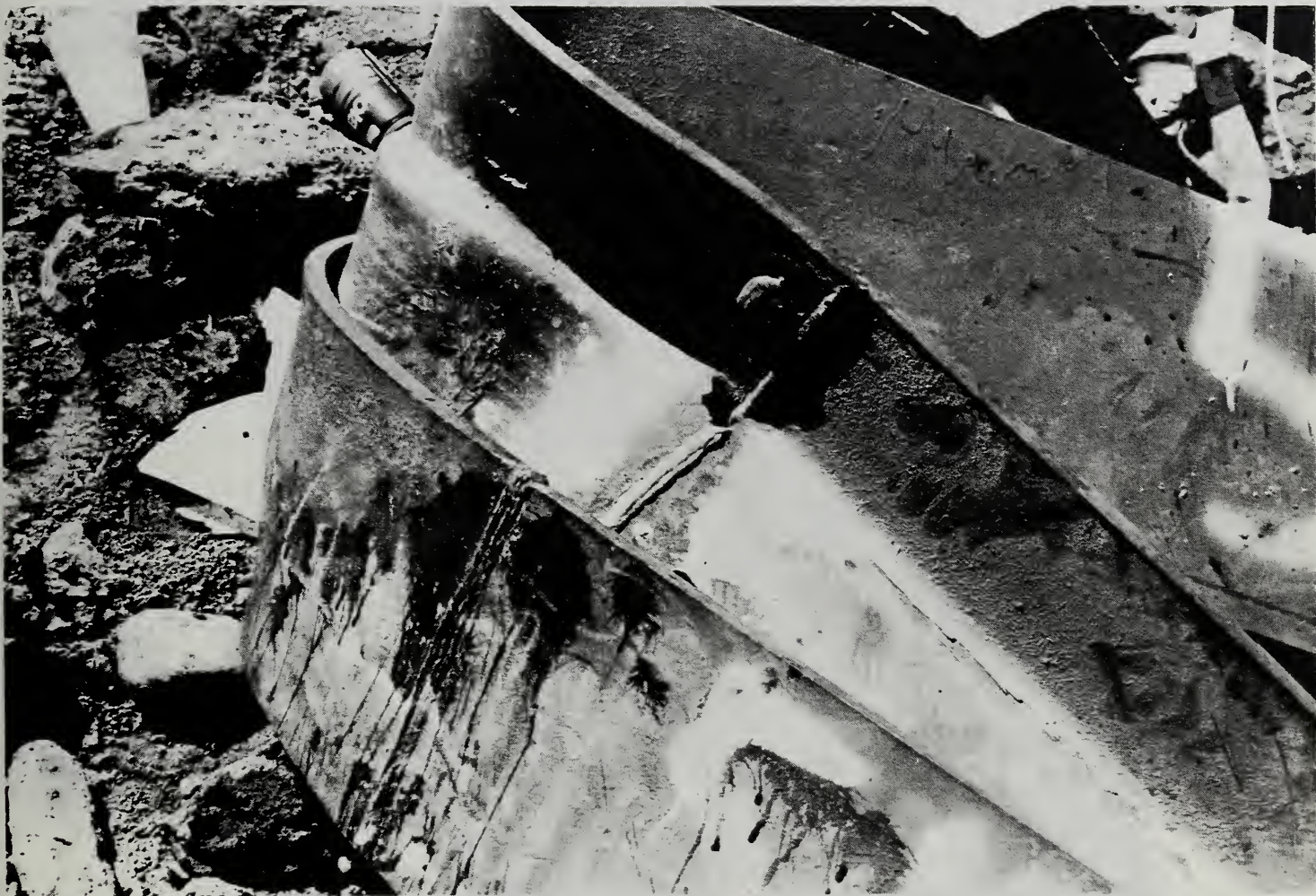
Figure 4.4.22 Deformation at column splice
