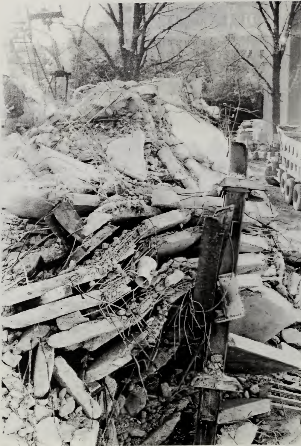
Figure 4.4.17 Broken floor slabs – View to the Southeast; column line H
