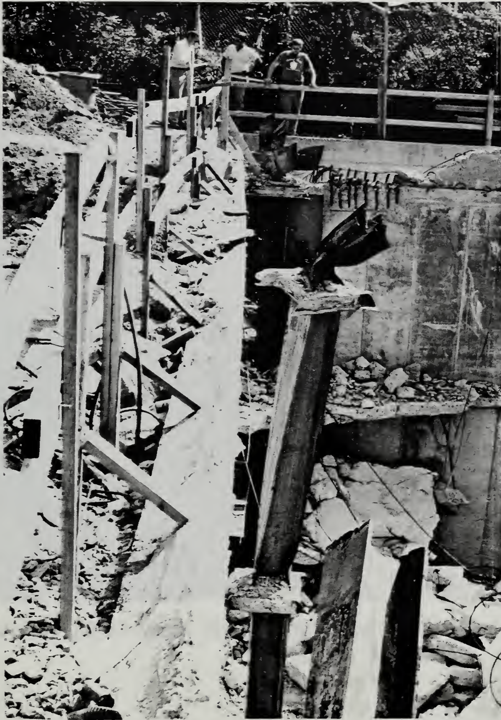
Figure 4.4.30 Basement wall on North side of East Tower – viewed from the West, July 22, 1987
