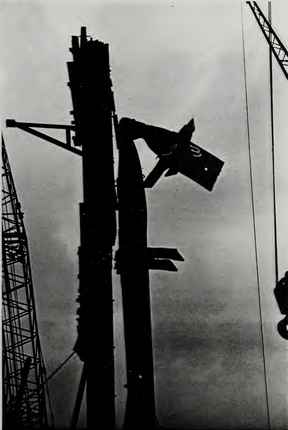
Figure 4.4.2 Column C3 bending about the strong axis - View to the East, shearwall on left
