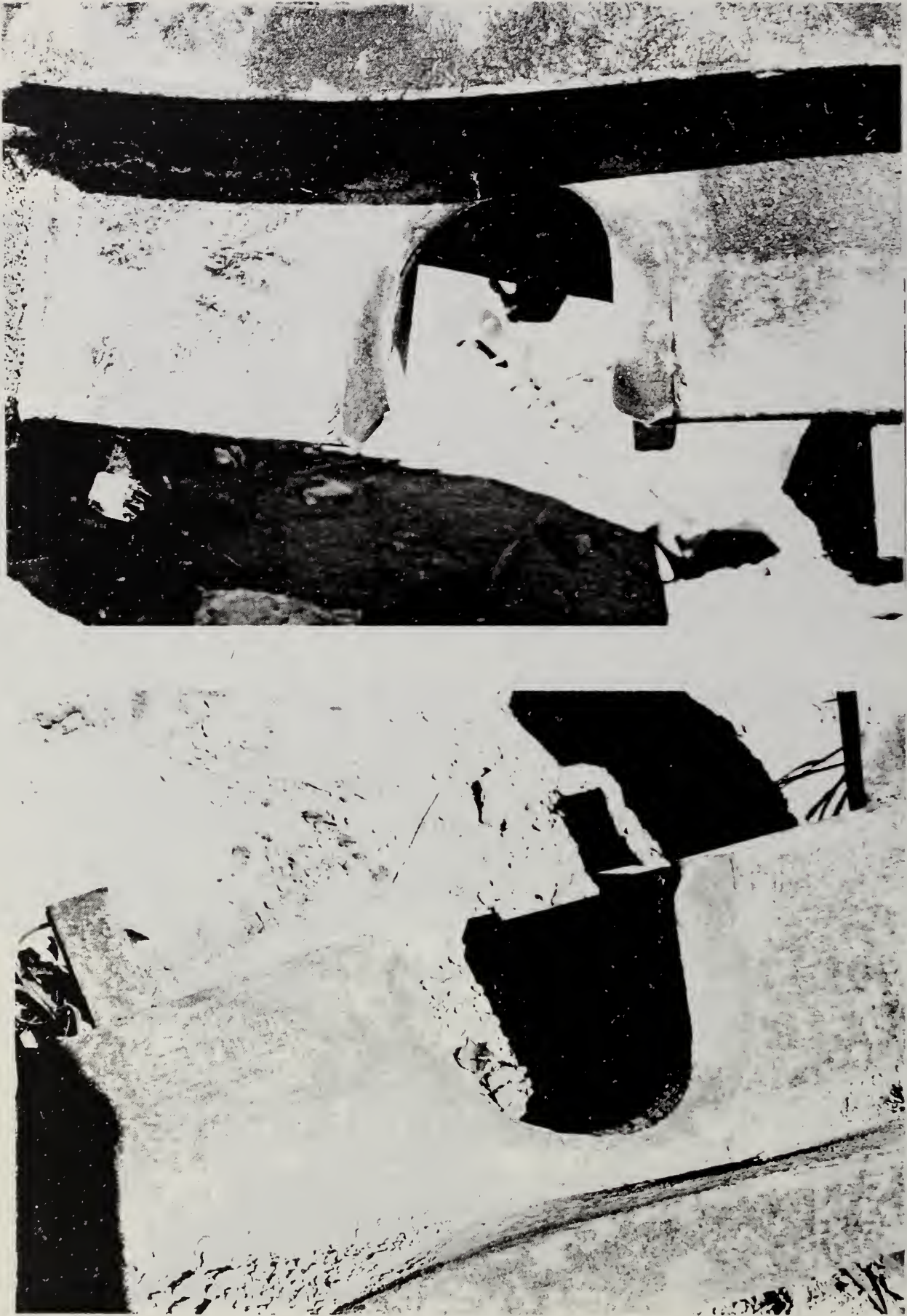
Figure 9.3.3 Indentations in underside of lifting angles, column E3.8, level 9
