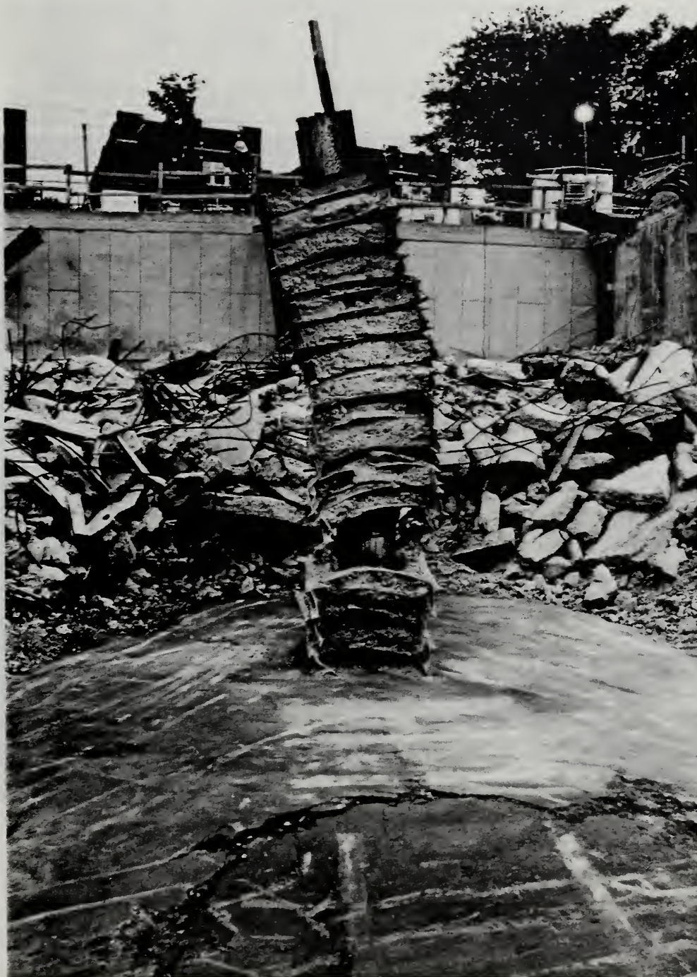
Figure 4.4.18 Deformation pattern of shearheads - column D10
