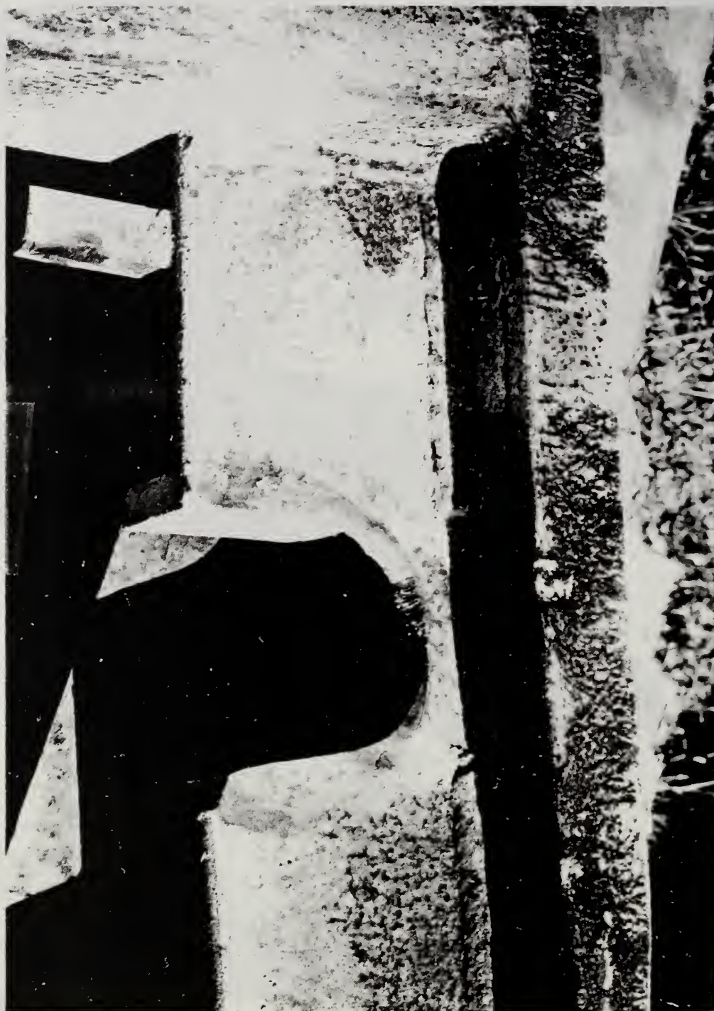
Figure 9.3.5 Indentation in underside of lifting angle, column E3.8, level 11
