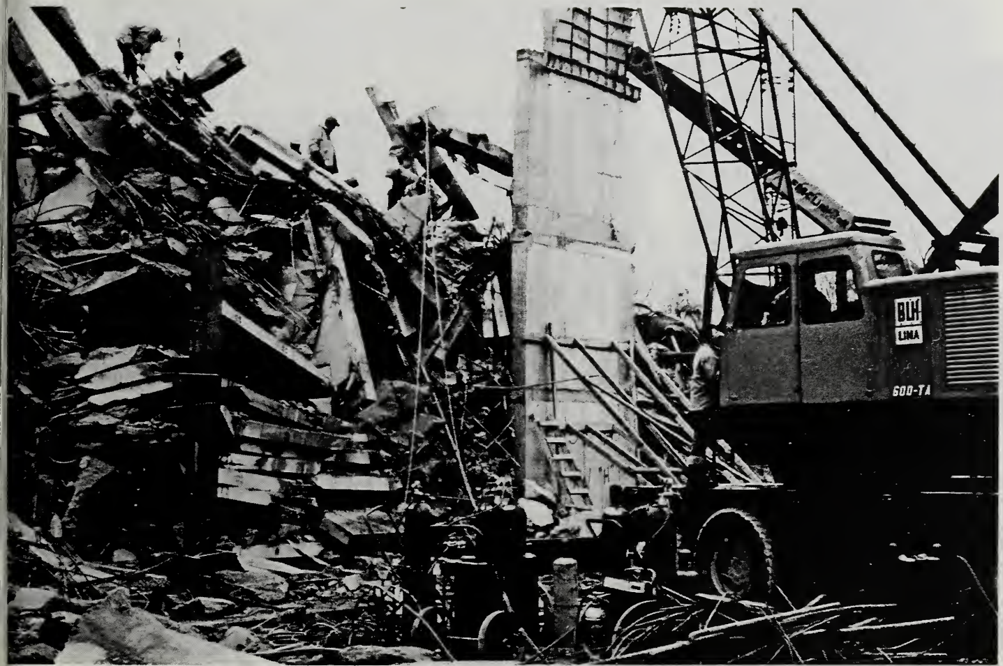
Figure 4.4.10 Lower level floor slabs in center portion of West tower – View to the Northeast
