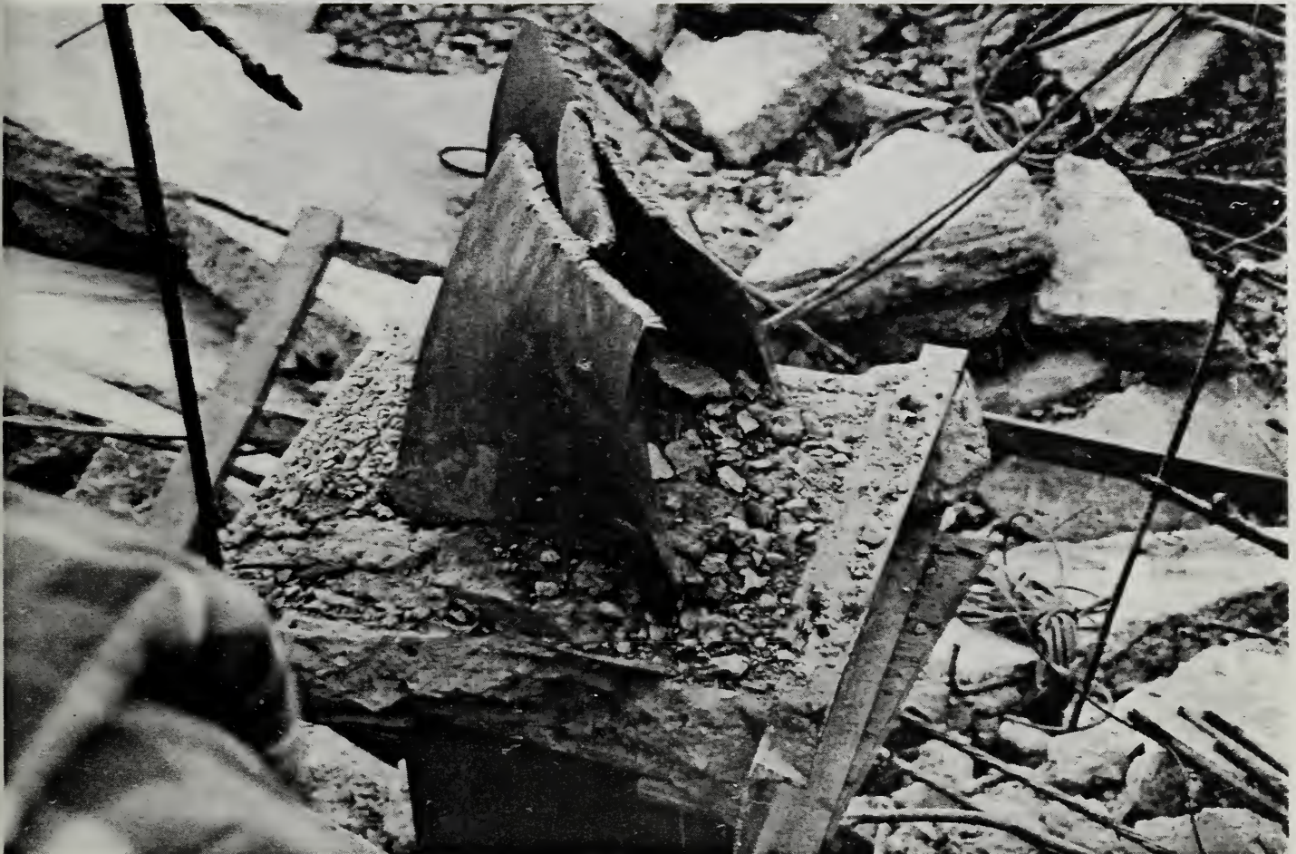
Figure 4.4.6 Twisting deformation of column in West tower
