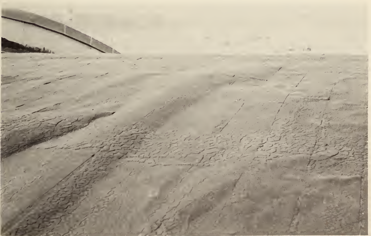
Figure 3. Blistering in Built-Up Membrane Roofing
