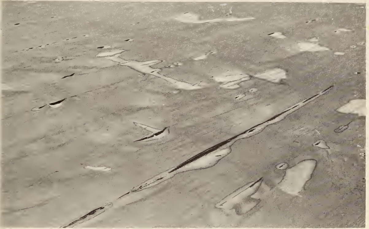
Figure 2. Membrane Wrinkling and Ridging (note water marks).
