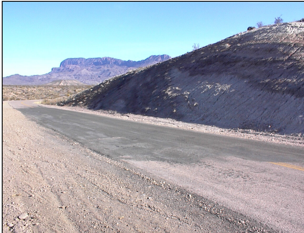
Figure 55.— This segment of Route 12 that crosses a stratum of Pen Clay has been repaired numerous times. Geefour silty clay occurs where the material, seen in the roadcut, is exposed at the surface. The high shrink-swell of the smectite clay deteriorates the pavement, necessitating continual maintenance of the road surface. The Chisos Mountains are in the background.
