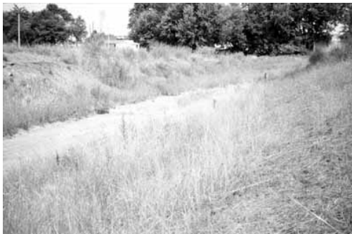
Poor coverage on upper slope
