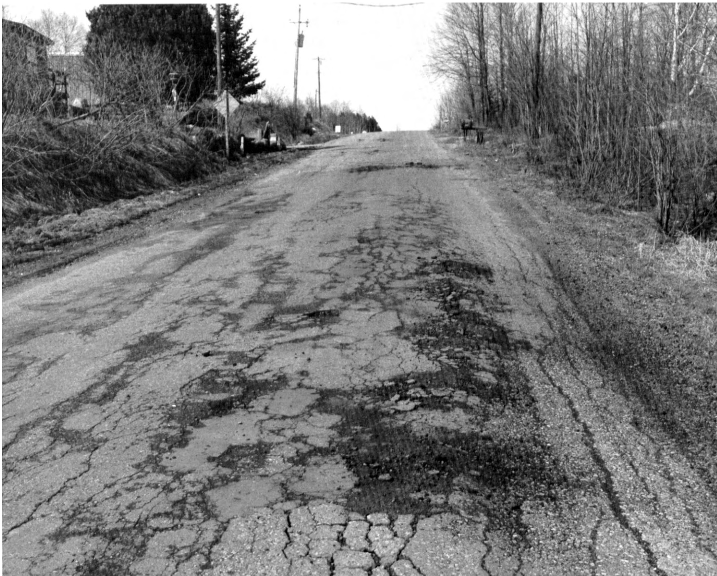
Figure 5.—Road damage caused by frost action in an area of Padus-Goodman complex, 1 to 6 percent slopes, stony.
