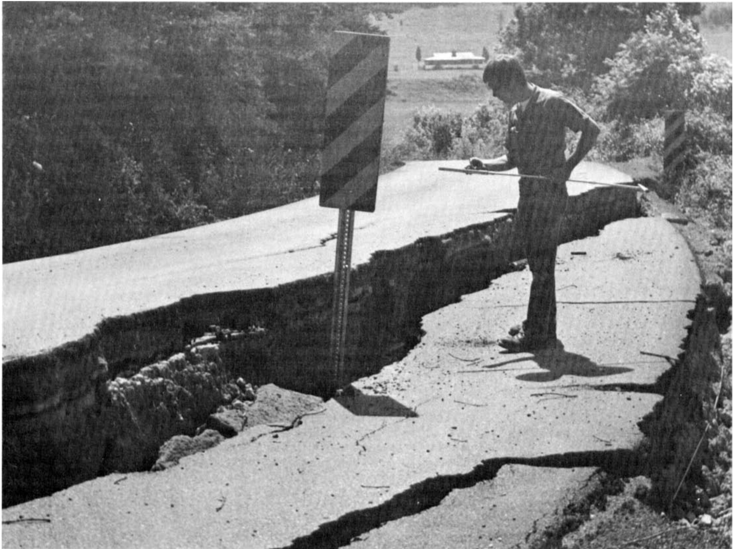
Figure 8.—Road failure due to slippage of Vandalia silt loam, 15 to 25 percent slopes.
