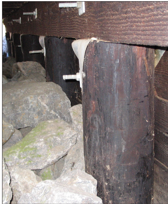
Figure 11. Pressure-treated round support piles used in applications such as this highway bridge are structurally critical and have a high decay hazard. They are treated to meet AWPA Use Category 4C.
