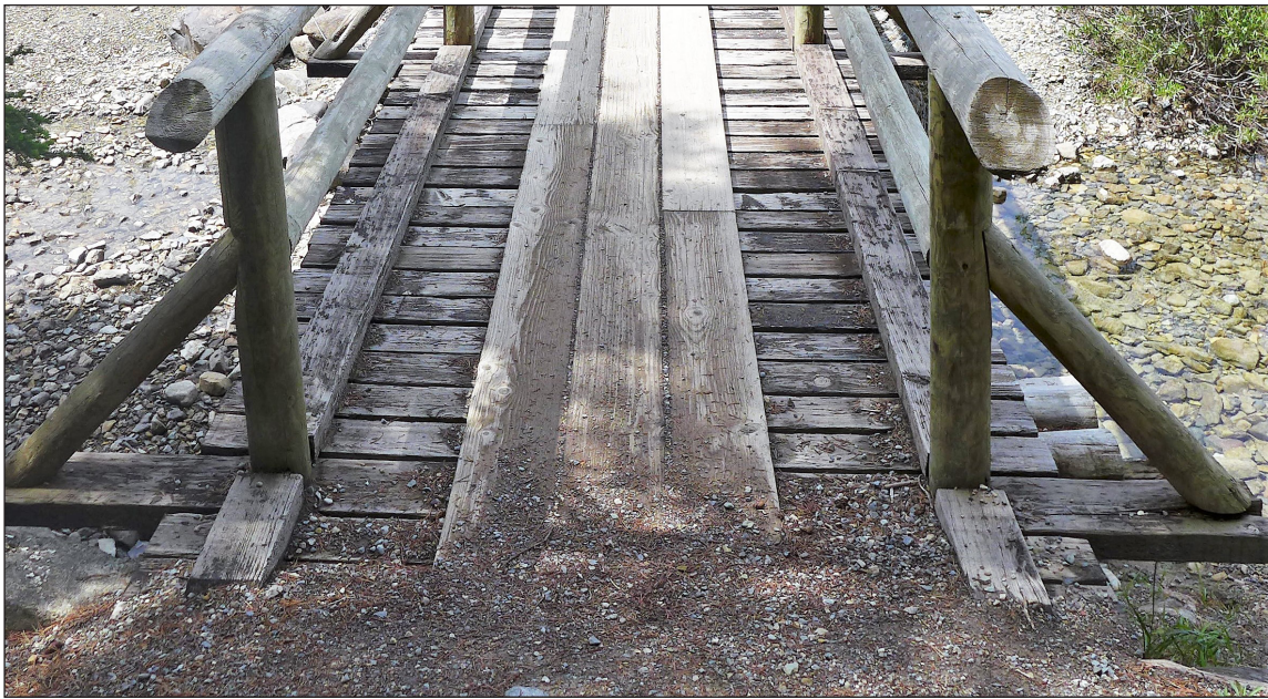
Figure 23. Gradual accumulation of dirt and other organic debris can create a ground contact decay hazard in portions of a structure that were originally above ground.
