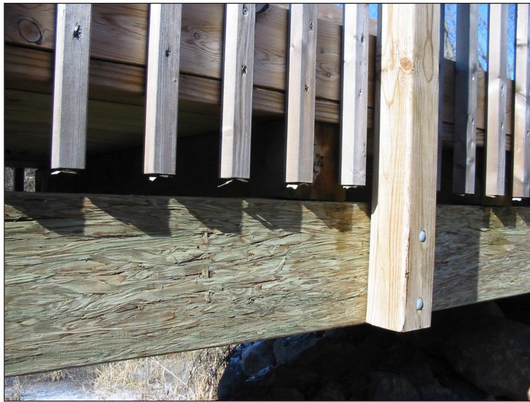
Figure 13. Pressure-treated parallel strand lumber (PSL) beams were used as supports for this trail bridge.
