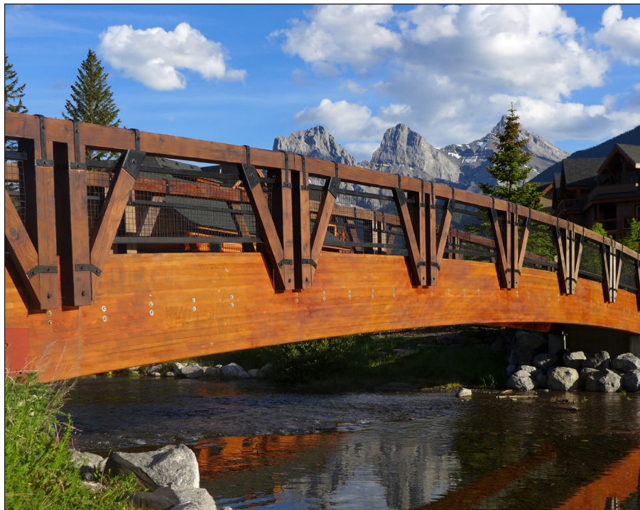
Figure 12. Pressure-treated glue-laminated timbers are frequently used to support bridges and in other applications with long spans and/or high strength requirements
