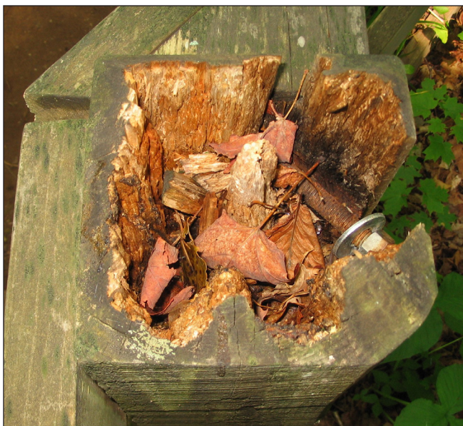
Figure 25. Sawn posts may contain poorly treated heartwood that is exposed if the post is cut to height after installation. If cutting to height is necessary, the exposed top should be coated with a field treatment preservative such as copper naphthenate.
