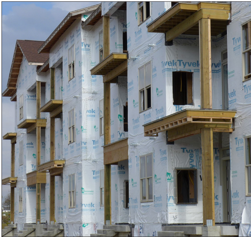
Figure 2. Lumber pressure-treated with waterborne preservatives is an important component of residential construction.
