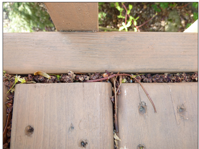
Figure 24. A deck construction design that covers the cut ends of the deck boards with a decorative skirt or fascia board. This practice allows organic debris to accumulate and trap moisture, which can increase the decay hazard and shorten the life of the structure.
