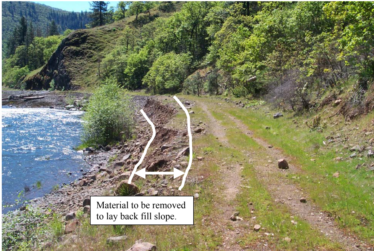
Figure 13: Actively eroding site about 3 miles downstream from Pitt. The upper 3 feet of existing railbed fill (as outlined in photo) would be laid back to a stable angle and revegetated to stabilize.
