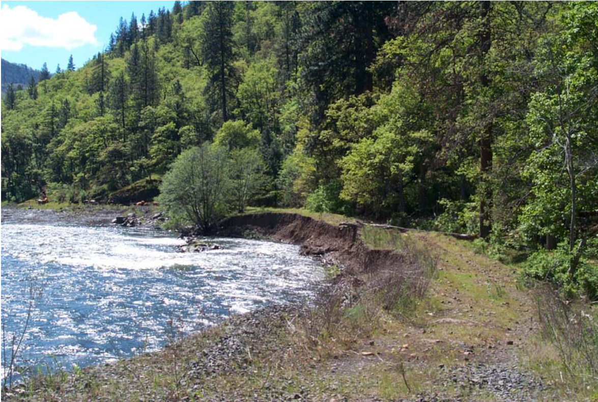
Figure 6: Erosion of the rail bed by the 1996 flood downstream of Pitt.
