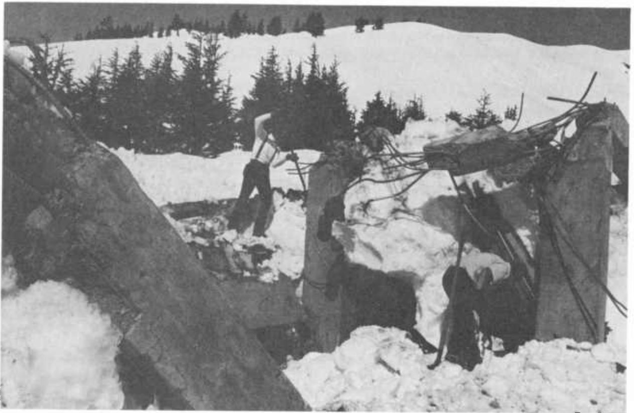
Figure 7.—Damage to the reinforced concrete base of a lift tower, Alyeska, Alaska, April 14, 1973. (Photo by O'Leary)
