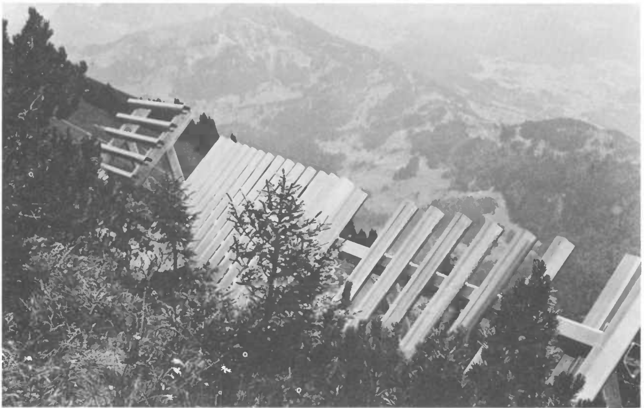
Figure 180.—Young trees on an avalanche slope in Switzerland with creep- and glide-control structures. (Photo by Frutiger)
