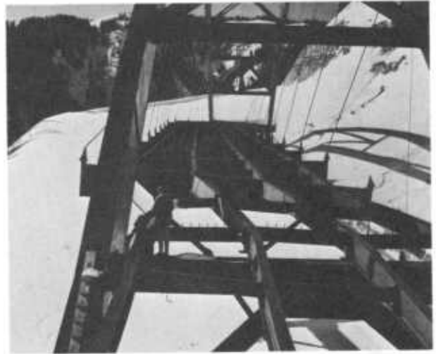
Figure 5.—Bent steel beams on bridge near Teton Pass, Wyo., testify to avalanche force, February 27, 1970. (Photo by Martinelli)
