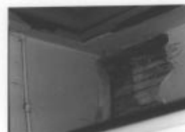
Water Damage Raymond High School
