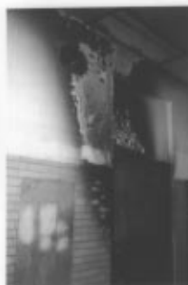
Unrepaired Fire Damage Chicago High School
