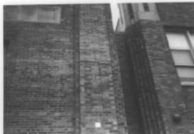
Structural Damage Chicago Elementary School
