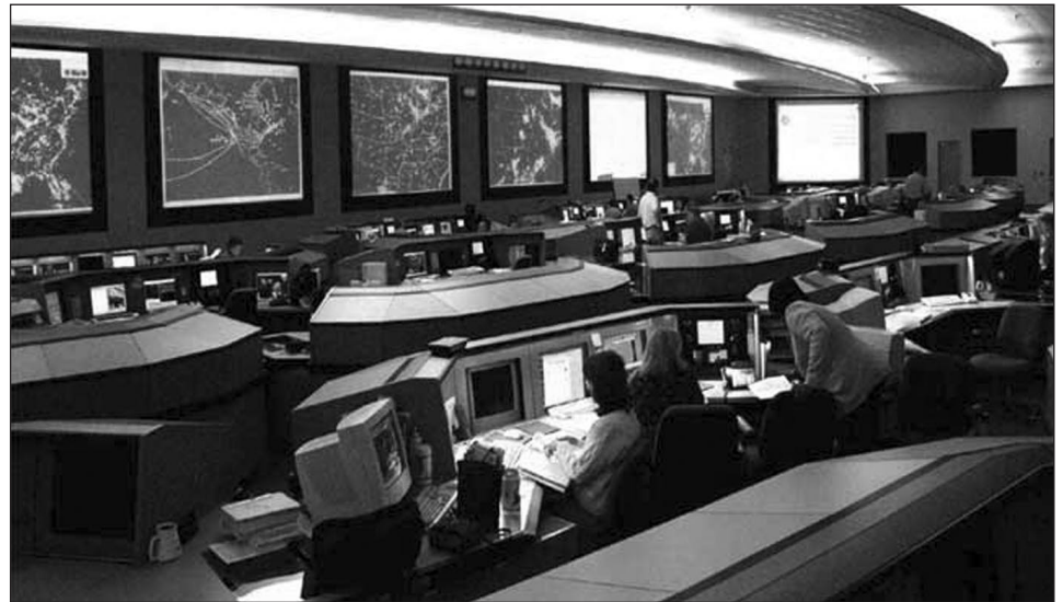
Figure 3: Air Traffic Control System Command Center
