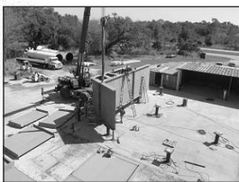
Atlas V West Coast Fixed Launch Platform Construction, Space Launch Complex 3E, Vandenberg Air Force Base, California
