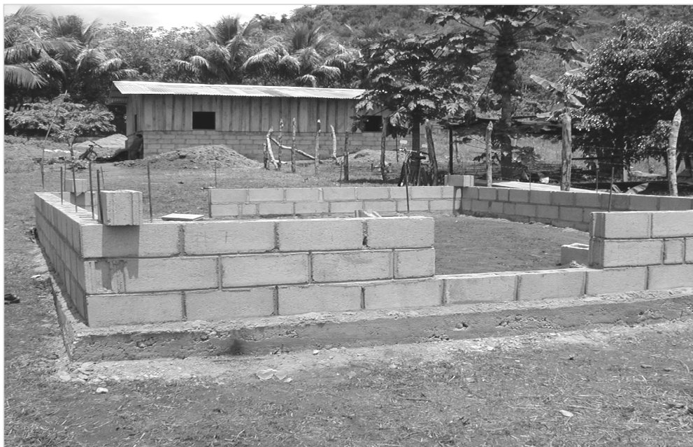
Figure 5: USAID-Assisted Construction Project to Build Permanent Housing in Rural Area of Honduras
