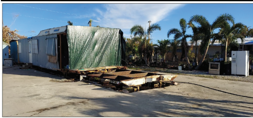
Figure 2: Hurricane Ian Damage to Home in Pine Island, Florida
