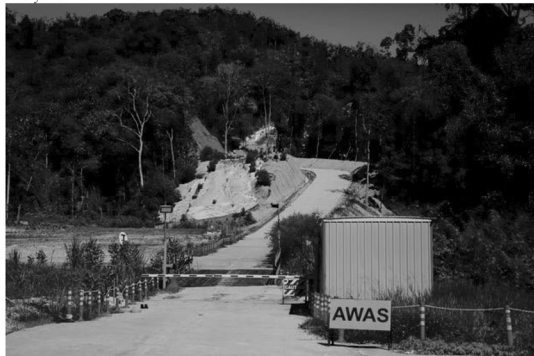
A tunnel approach for a $16 billion rail link China agreed to build for Malaysia. The government that took over in Malaysia last year has suspended the project.
