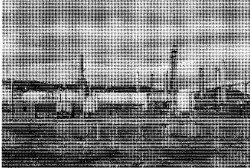
The Beaver Creek plant. Natural gas has been a bonanza to Wyoming, which gave President Trump his biggest margin of victory in the election.
