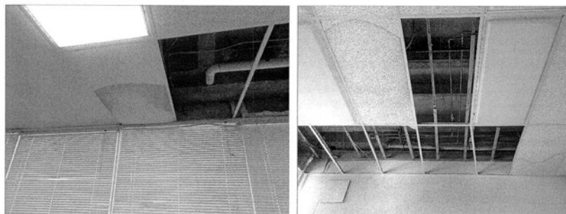
Figure 5: Damaged or Removed Classroom Ceiling Tiles Due to Leaks in Recently-Installed Roofs
