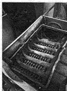
#2 cleaned flue passag
