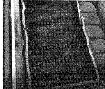
sooted flue passage inside boiler section
