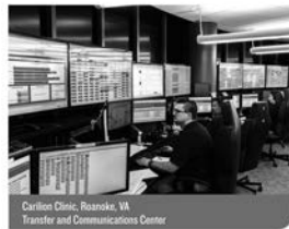
Carilion Clinic, Roanoke, VA Transfer and Communications Center
