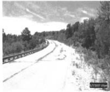
Hualapai Reservation. Example of deteriorated road pavement conditions. Provided courtesy of the Hualapai Tribe.
