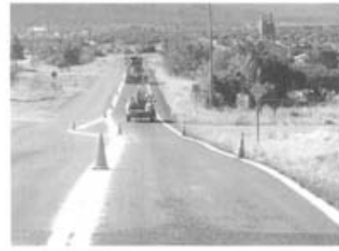
Fort Apache Reservation. Example of a striping project. Provided courtesy of BIA Fort Apache Agency
