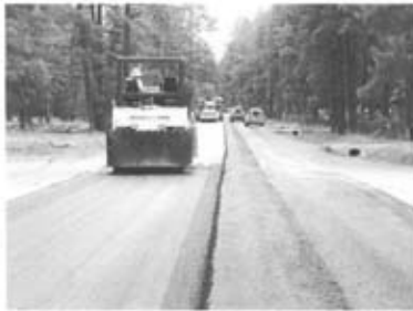
Fort Apache Reservation. Example of a reconstructed street due to lack of routine maintenance. Provided courtesy of BIA Fort Apache Agency.
