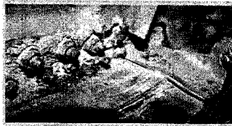
Close-Up Picture of Severe Strut Corrosion
